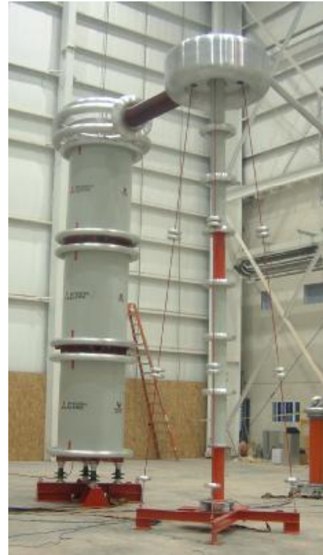
675kV, 3375kVA, Cylinder Type Reactors for Onsite Testing of GIS
